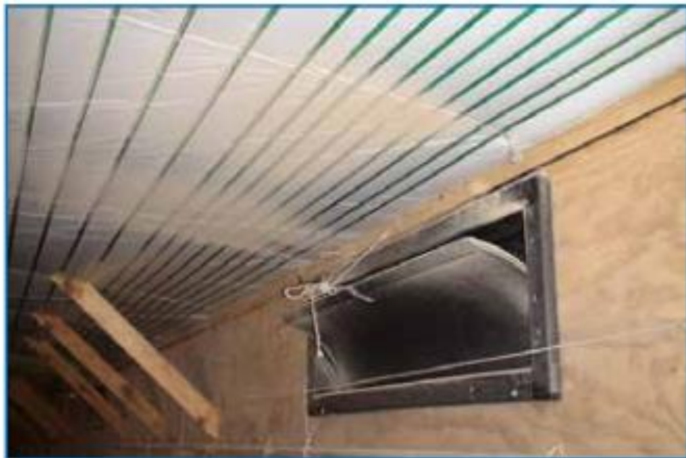
Figure 36: Example of a good quality air inlet.
